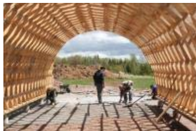
Workers lay the floor for the new building at the Ross Creek Centre for the Arts. (GLEN PARKER)
